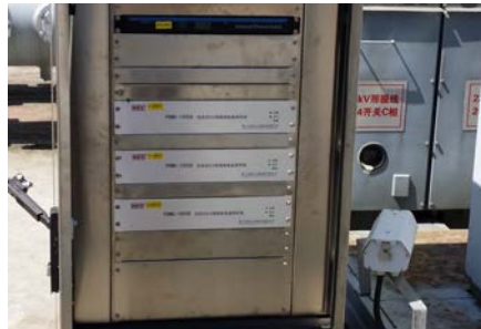
Data Acquisition Unit (DAU)
